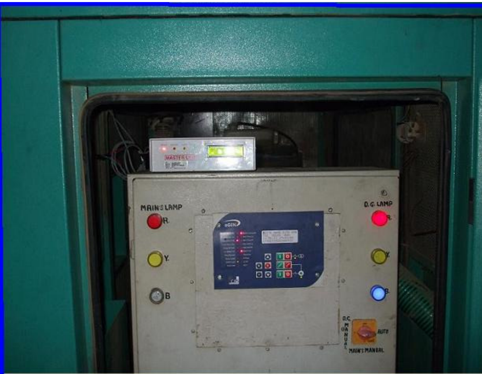
View of Real working Automatic D.G. operator BSNL site.
